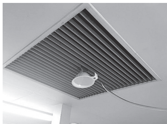
Fig.2 Which the tip of the hose of the dust sampler is installed at the exhaust port
